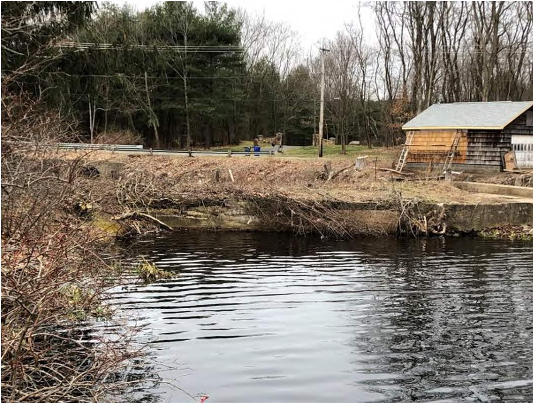
Photo 3 – Upstream view of embankment retaining wall cracks and spalling
