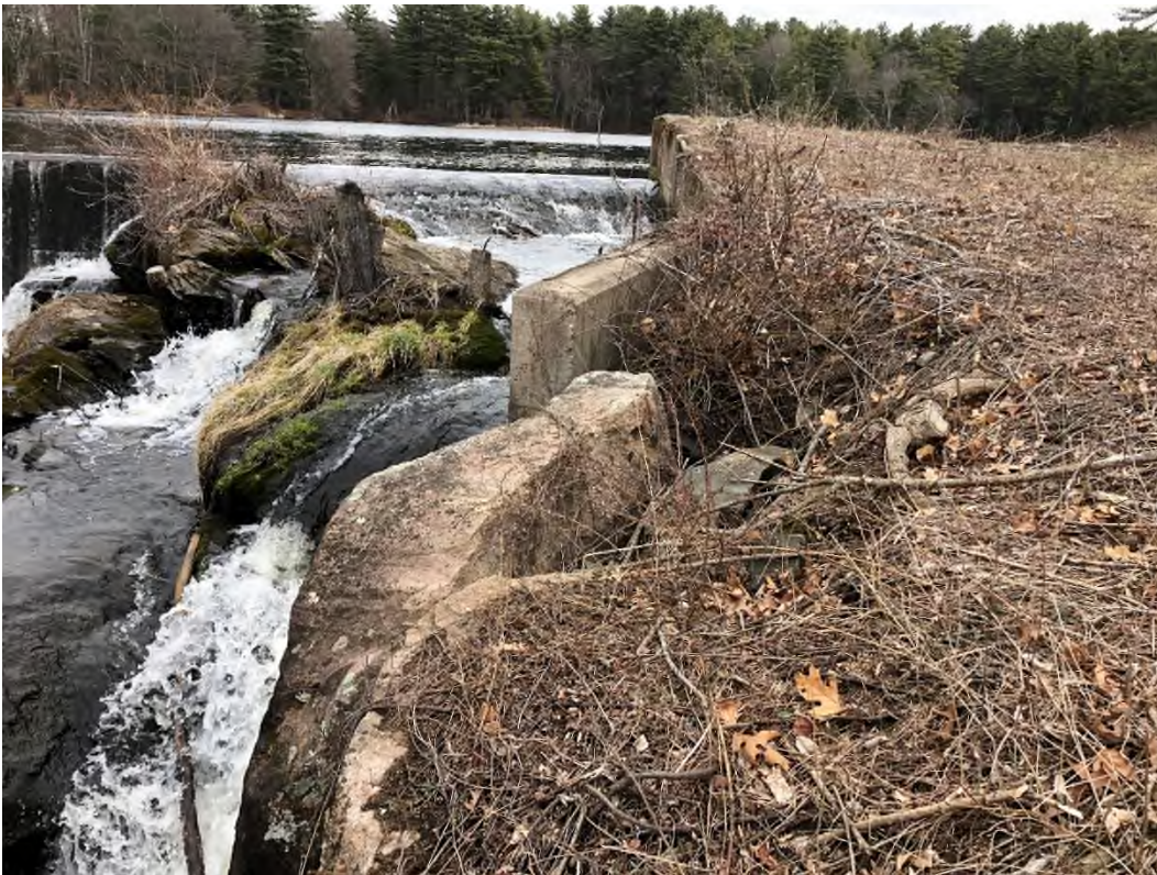
Photo 14 – Left side of spillway with erosion behind left downstream training wall
