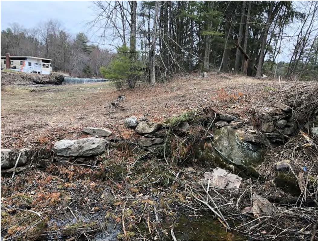
Photo 13 – Downstream stone retaining wall at discharge channel to the right of low level outlet
