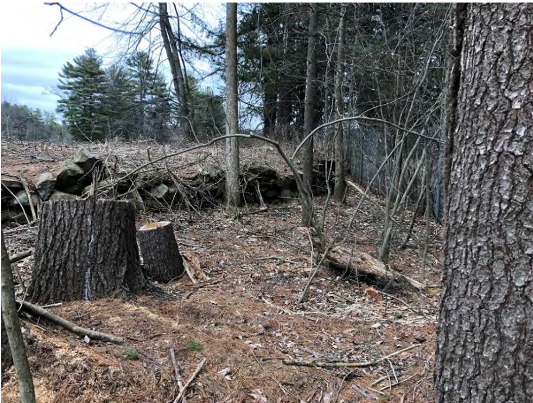
Photo 14 – Stone masonry wall on downstream slope to the left of the low-level outlet Forge Pond Dike, Granby Date of Inspection: March 23, 2020
