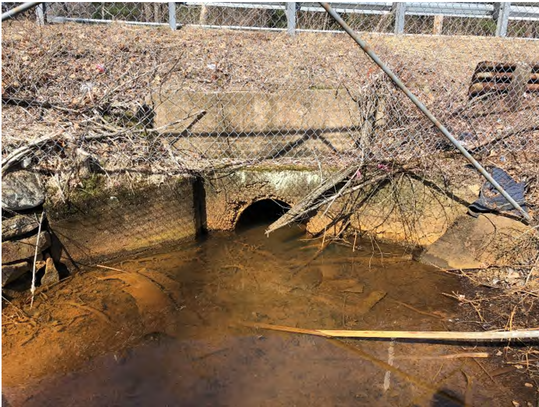
Photo 20 – Upstream end of culvert passing under School Street downstream of low-level outlet
