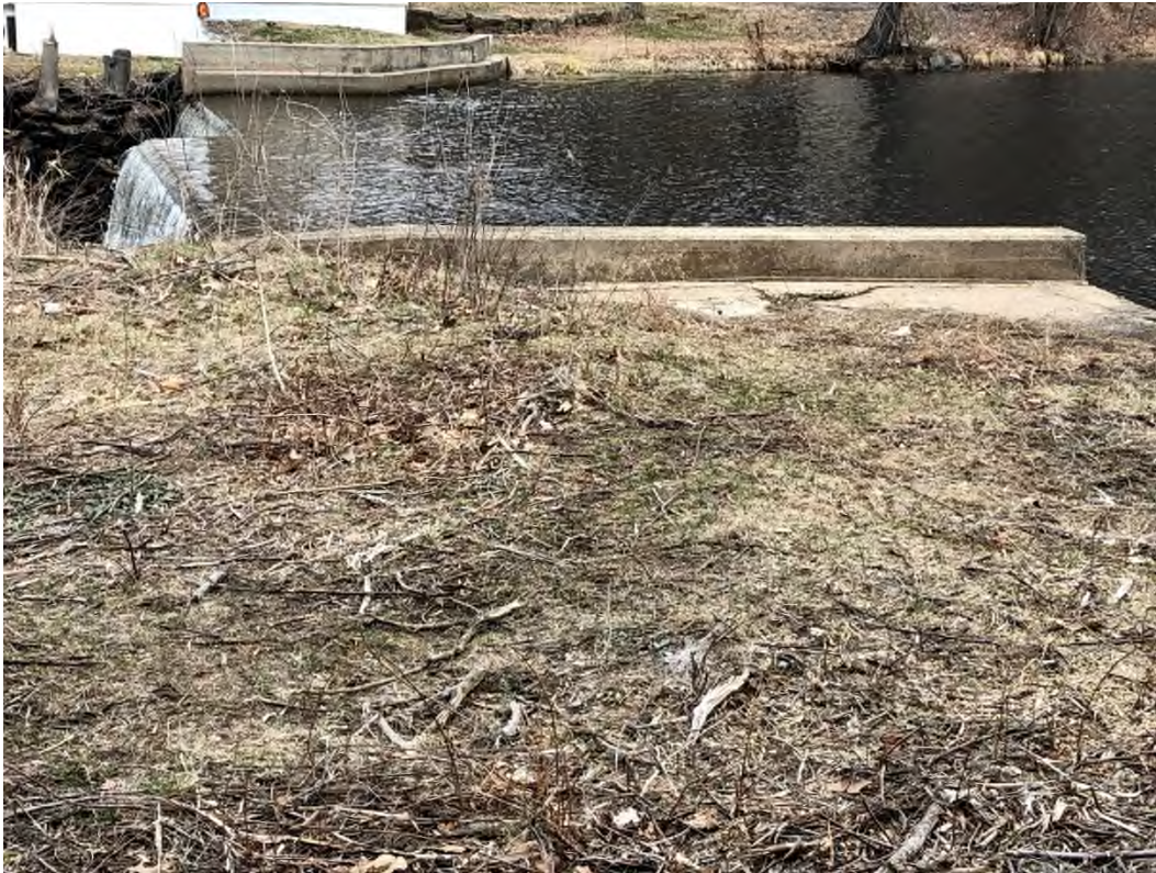
Photo 7 – Back of left training wall and spillway crest viewed from left side
