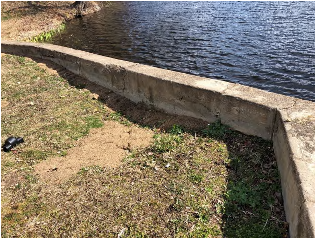
Photo 12 – Settlement and rotting stump behind right upstream spillway training wall
