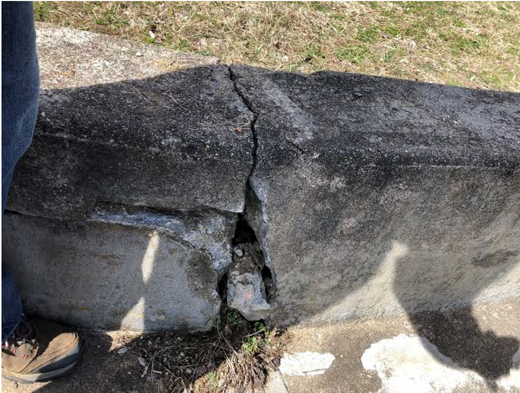
Photo 17 - Deteriorating concrete on upstream face of right spillway training wall
