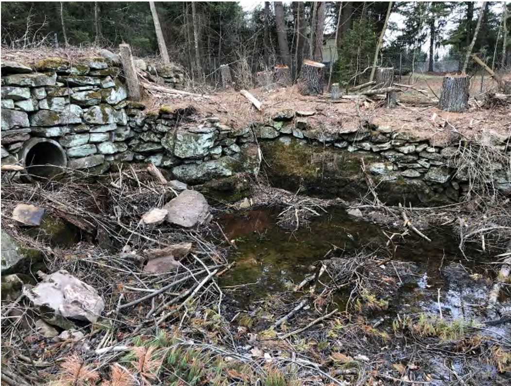
Photo 12 – Stone masonry retaining wall at discharge channel to the left of low level outlet
