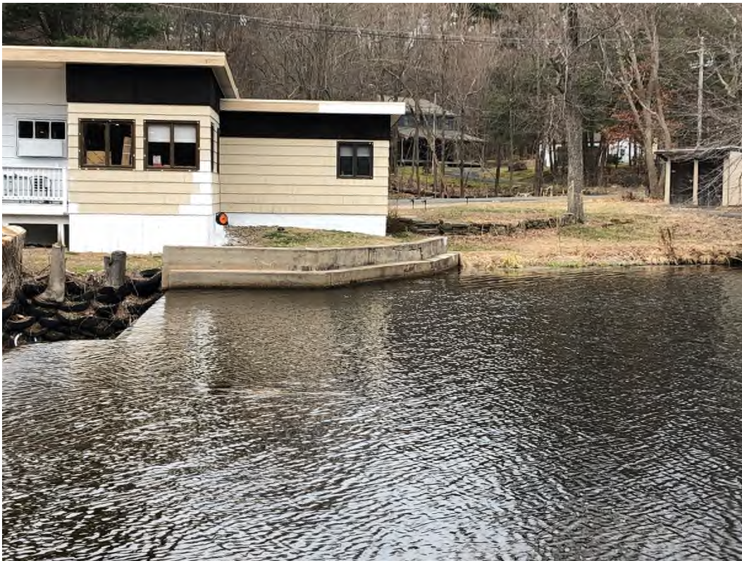
Photo 16 – Spillway crest, deteriorating concrete on right training wall and upstream retaining wall
