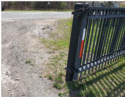
Image 2: Existing conditions showing encroachment on the grass and ponding at edges of entrance driveway.
