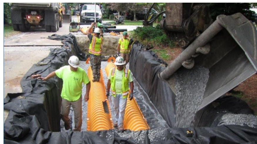
Image 2: Installation of a subsurface infiltration system in Narragansett, RI (image source: RIDOT Linear Stormwater Manual)
